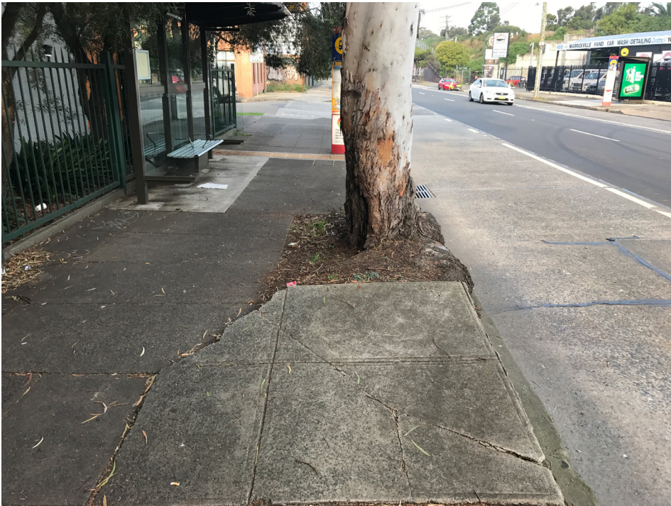
Marrickville Road's north side, existing bus stop. Footpath damaged by existing Eucalyptus Mannifera (high retention value).
